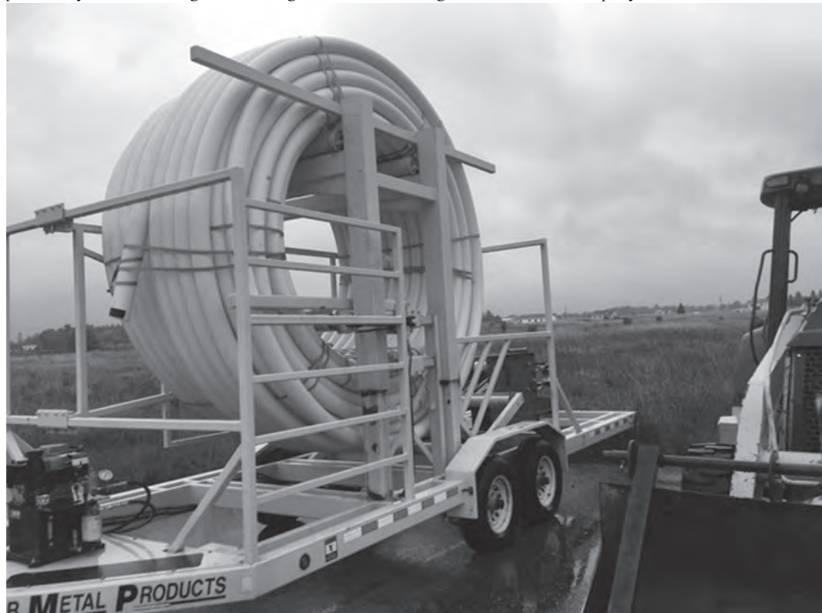
Some of the equipment DTE and Roese Construction Company are using to bring natural gas into the Odenaang Housing site in Sault Ste. Marie, Mich. The companies are installing the main lines along Seymour just south of the Sault city limits into the Odenaang Housing area.
