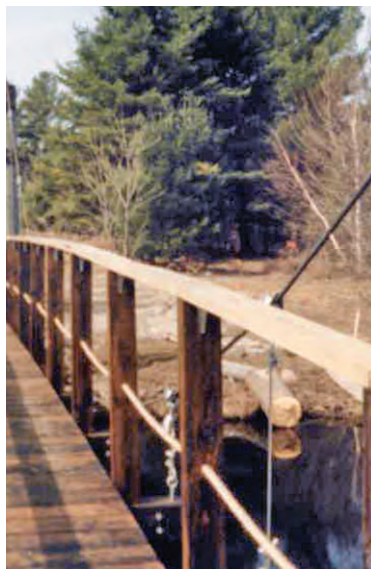
Originally built in the 1980s during development of the 2,000-mile long national hiking trail, the Naomikong "Mini-Mac" Bridge had been built to mimic the look of the Mackinac Bridge that spans the Straits of Mackinac.
