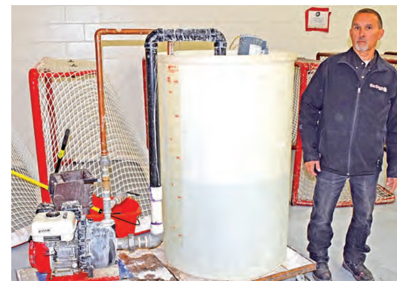
Operations Manager Hutte with the reservoir apparatus used to mix the paint and water. To the left of the reservoir is the pump used to force paint through the hose and spray boom used to apply the white paint on the ice surface.
