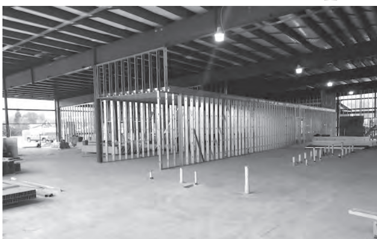
Above is a look at interior construction of the classroom addition at JKL Bahweting School. The project is due to be complete in two months.
