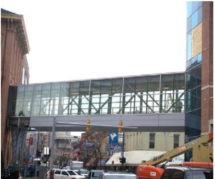
Greektown Casino's new attached parking structure is more convenient for patrons. Pictured is the pedestrian walkway from the casino to the parking garage.
