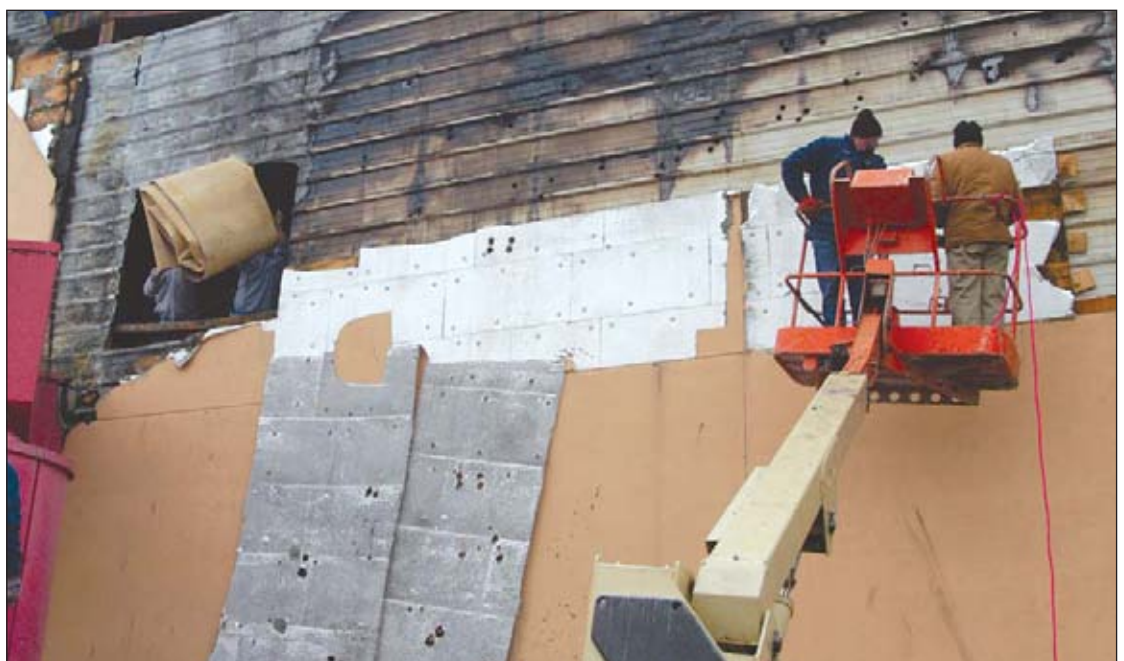
Clean up crews throw the trash out of the second floor of the Sault casino and remove the damaged siding and insulation where an electrical fire started in February, 2004. The fire caused extensive smoke and water damage to part of the casino which was completely remodeled and reopened June 2005. Photo by Alan Kamuda
