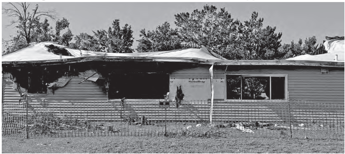
Duplex on Shadow Wood Lane in Kincheloe, Mich., destroyed by fire on Sept. 1. No lives lost, no injuries.
