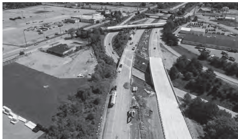
The $60 million project to replace pavement on I-496 is the first to be funded through Whitmer's Rebuilding Michigan program.
