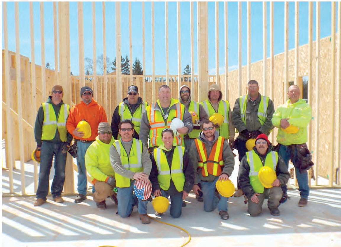
The Force Account construction crew working on the elder complex in May 2017. The 14 crew members (one is missing from photo) are all tribal members from the Sault, St. Ignace, Manistique and Cheboygan.
