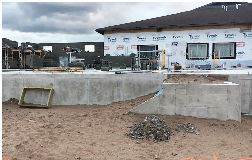
Renovations added a two-car garage, conference room, visitation room, office, temporary holding cells and secure access to Tribal Court.
