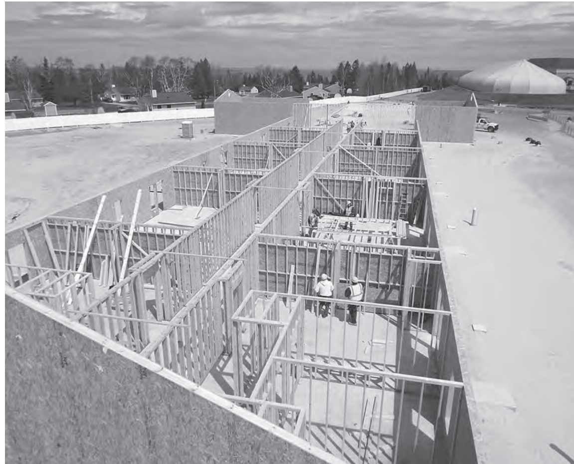
The 5-acre Red Lightning Woman Elder Complex located in St. Ignace — named in honor of late Sault Tribe Housing Commissioner Shirley Goudreau — is now under construction.
