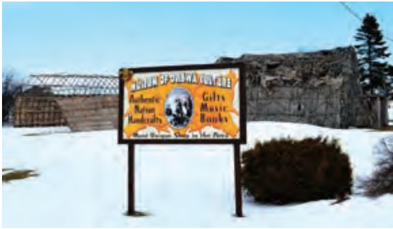
A new longhouse (left) is being built on the grounds of the Museum of Ojibwa Culture in St. Ignace to replace the one that is falling apart.
