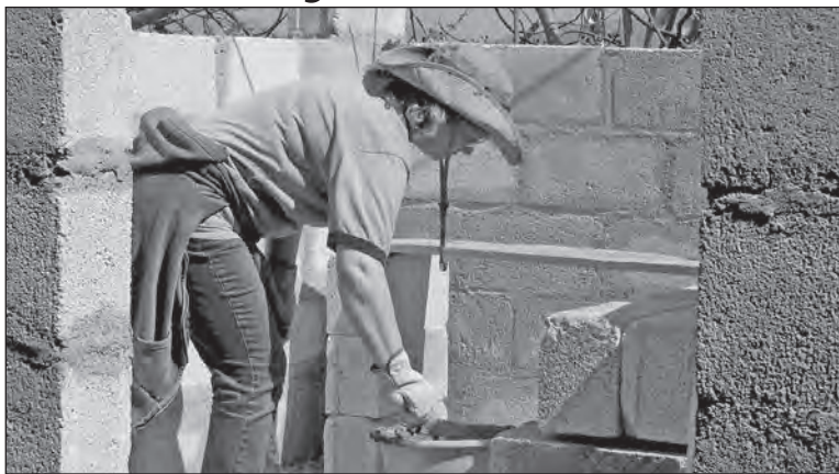
Pat Pyle works to help build a local family a new home.
