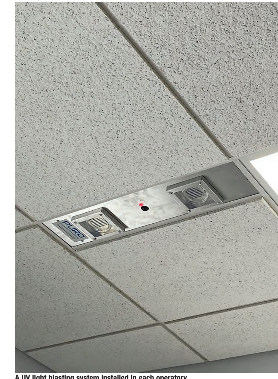
A UV light blasting system installed in each operatory.
