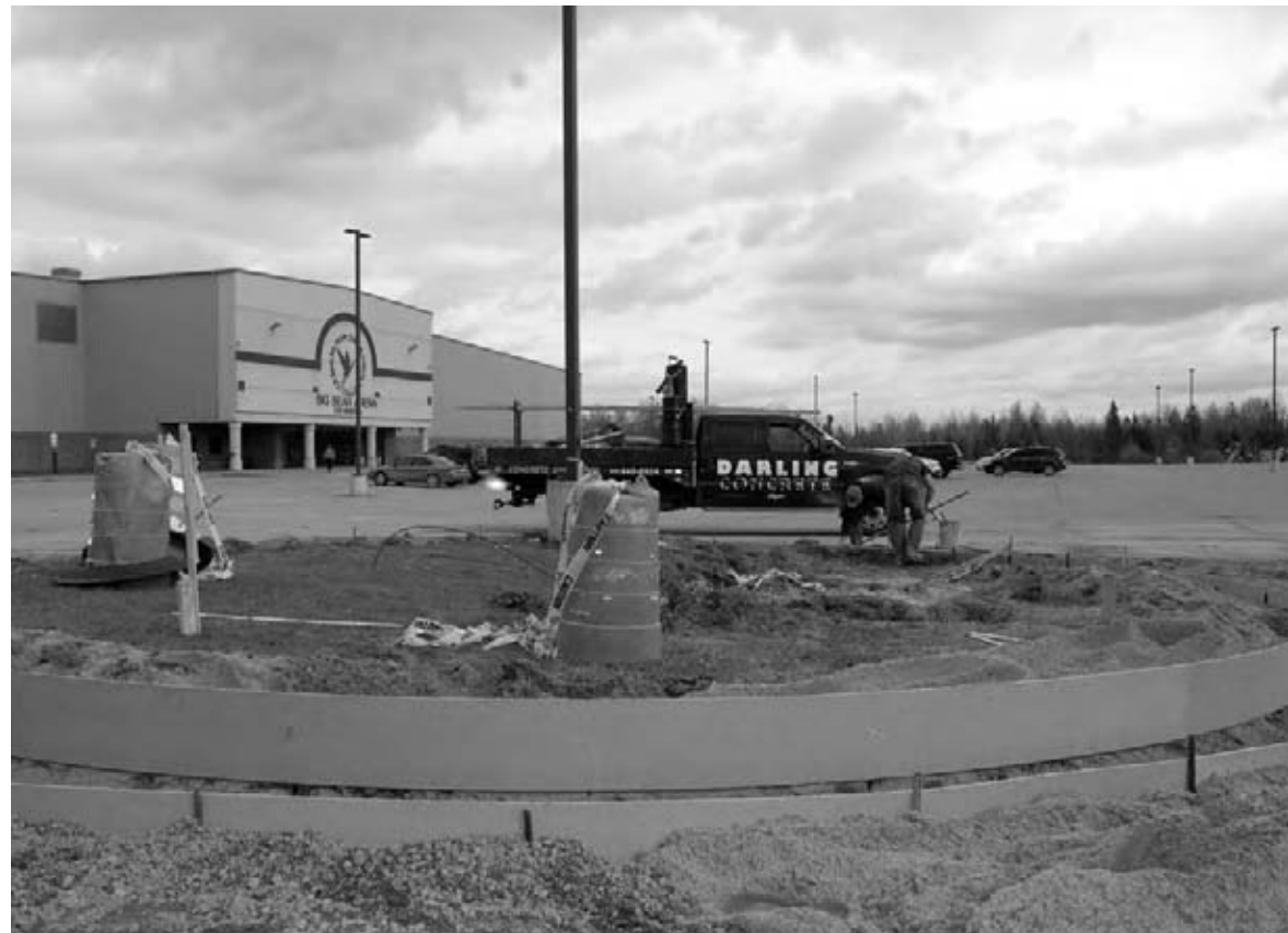
Photo by Brenda Austin Sault Tribe Transportation recently completed reconstruction of the entrances at Big Bear and Enrollment Department facilities in Sault Ste. Marie. Key upgrades included new culverts, asphalt, curb and gutter. It is anticipated these upgrades will promote safer access to services offered at these facilities.
