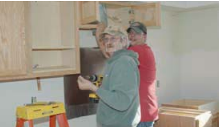
Left: Fred Albon and Wayne McKerchie, carpenters, installing a range hood in one of the rental housing units in St. Ignace.
