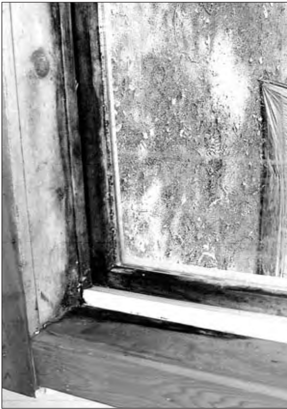
The rotting window, above, is an example of where there is heat loss and the weatherization program can assist.
